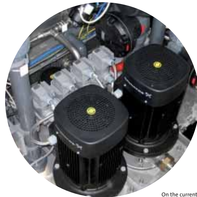
On the current ECM installations, Extrude Hone VMB is now changing all pumps to immersion pumps of the MTRI series, which also feature a stainless steel head.
